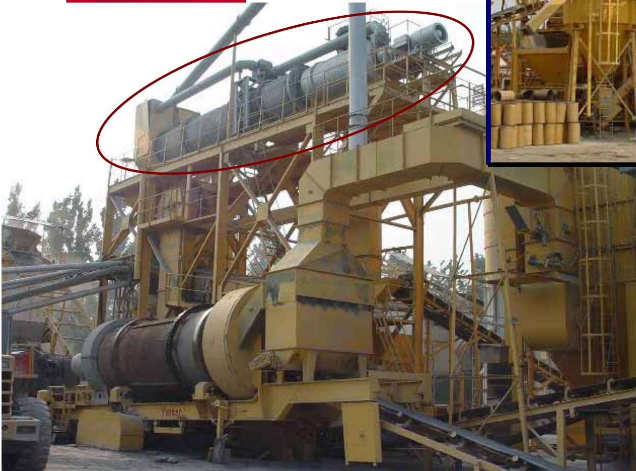
Batch Plant with double drum in Beijing
